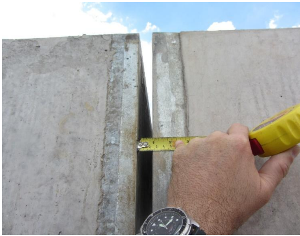
Alstom — Depot, Line 15 São Paulo
